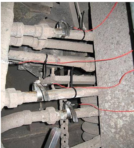
Acousto ultrasonic-echo taphole inspection
